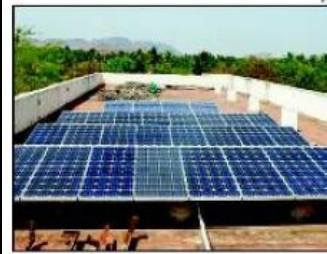
Pilot project is looking at generating 500kW of power through rooftop solar photovoltaic cells
