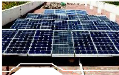
Solar panels atop a building
